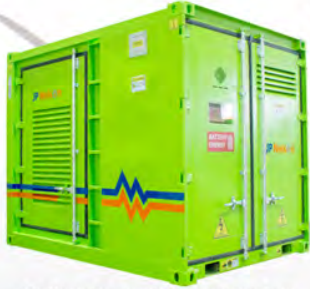
Battery Energy Storage System
